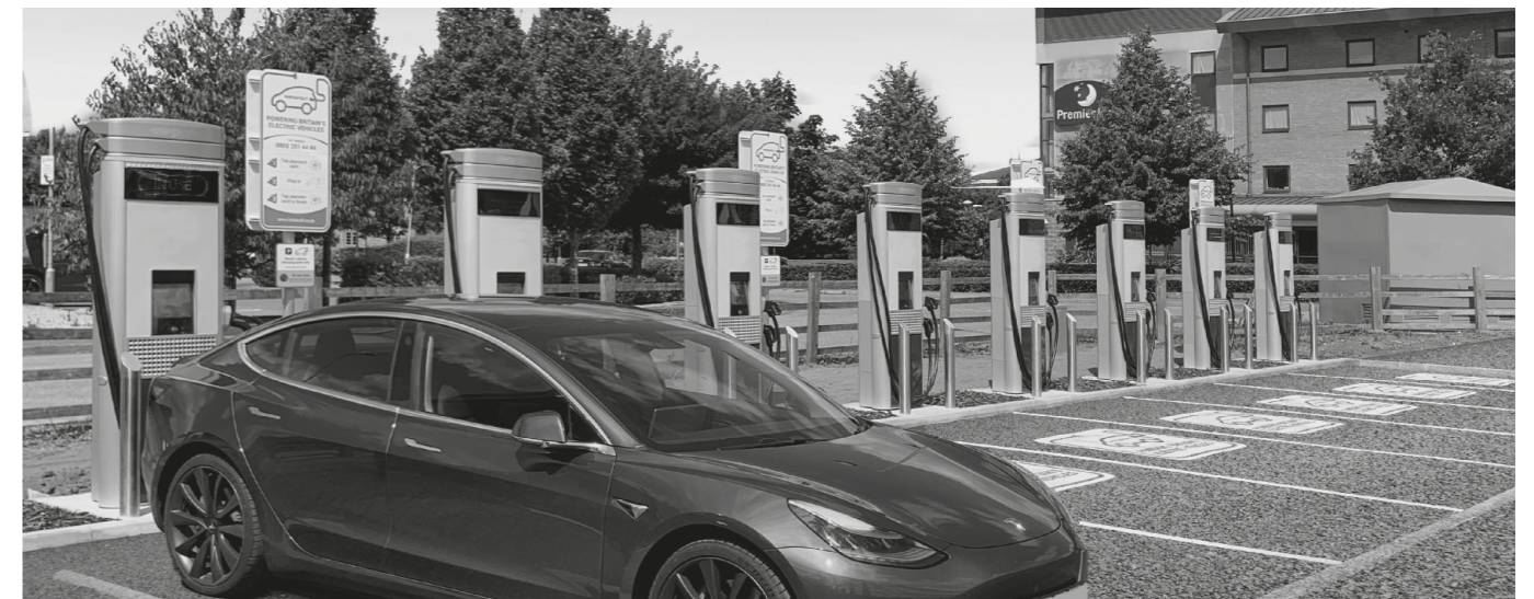
Electric Vehicle Charging
